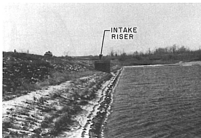
Figure 1. Pre-Repair Lake Below Intake Riser (Normal Pool) Control on Upstream Slope of Dam
